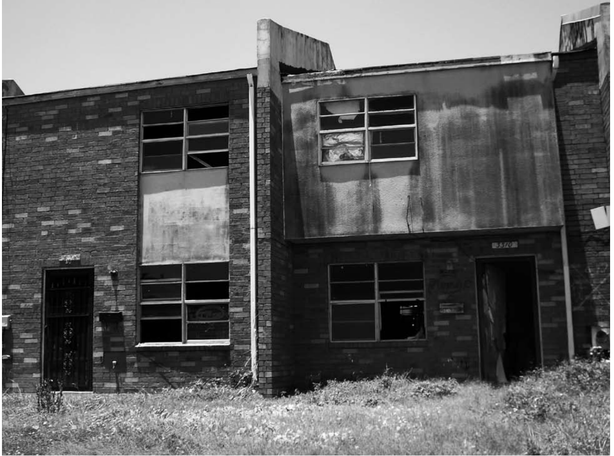
Gutted remnants of St. Bernard Housing structures hit by Hurricane Katrina
